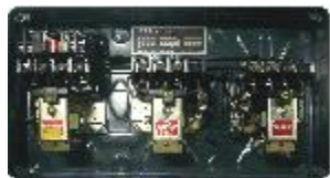
Interior View of MK1 SASD
